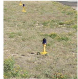
Blue Taxiway Edge Light
