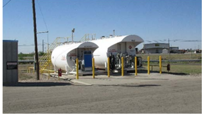
Christian Aero LLC Self-Service Fuel Tanks
